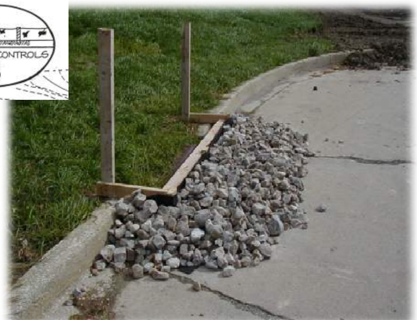
Curb Inlet Protection
