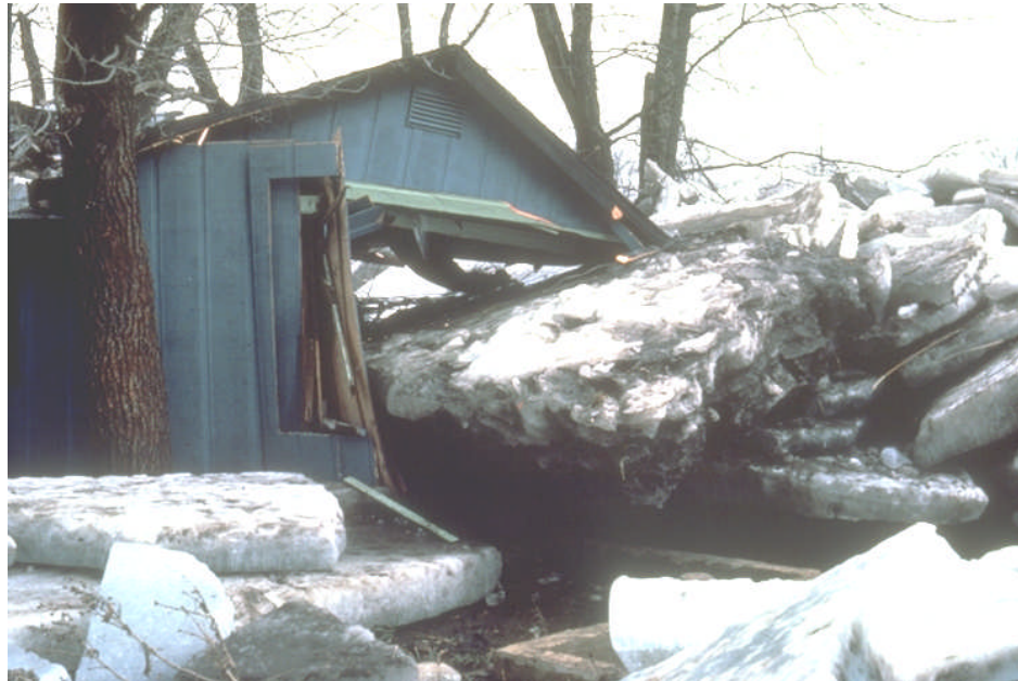
Figure 2-8: Ice floes and other large items of debris can crush a house (Kankakee River, 1985)
