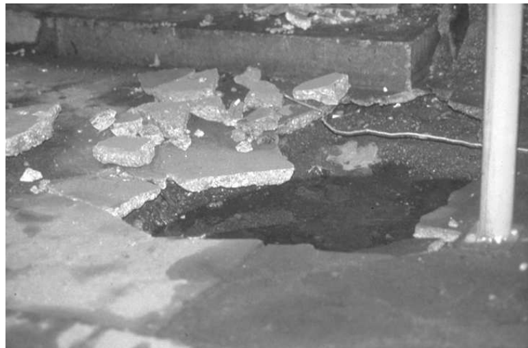
Figure 2-10: This basement floor broke from hydrostatic pressure
