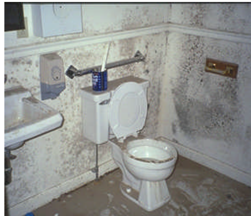
Figure 2-6: Post-flood silt, mold, and mildew
