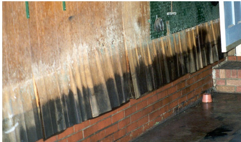
Figure 2-11: Prolonged exposure to water and “wicking” can destroy wood and gypsum walls.
