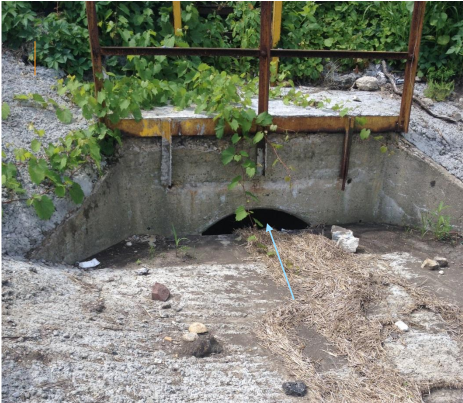
5 Storm Sewer Inlet (Neglected due to small opening)
