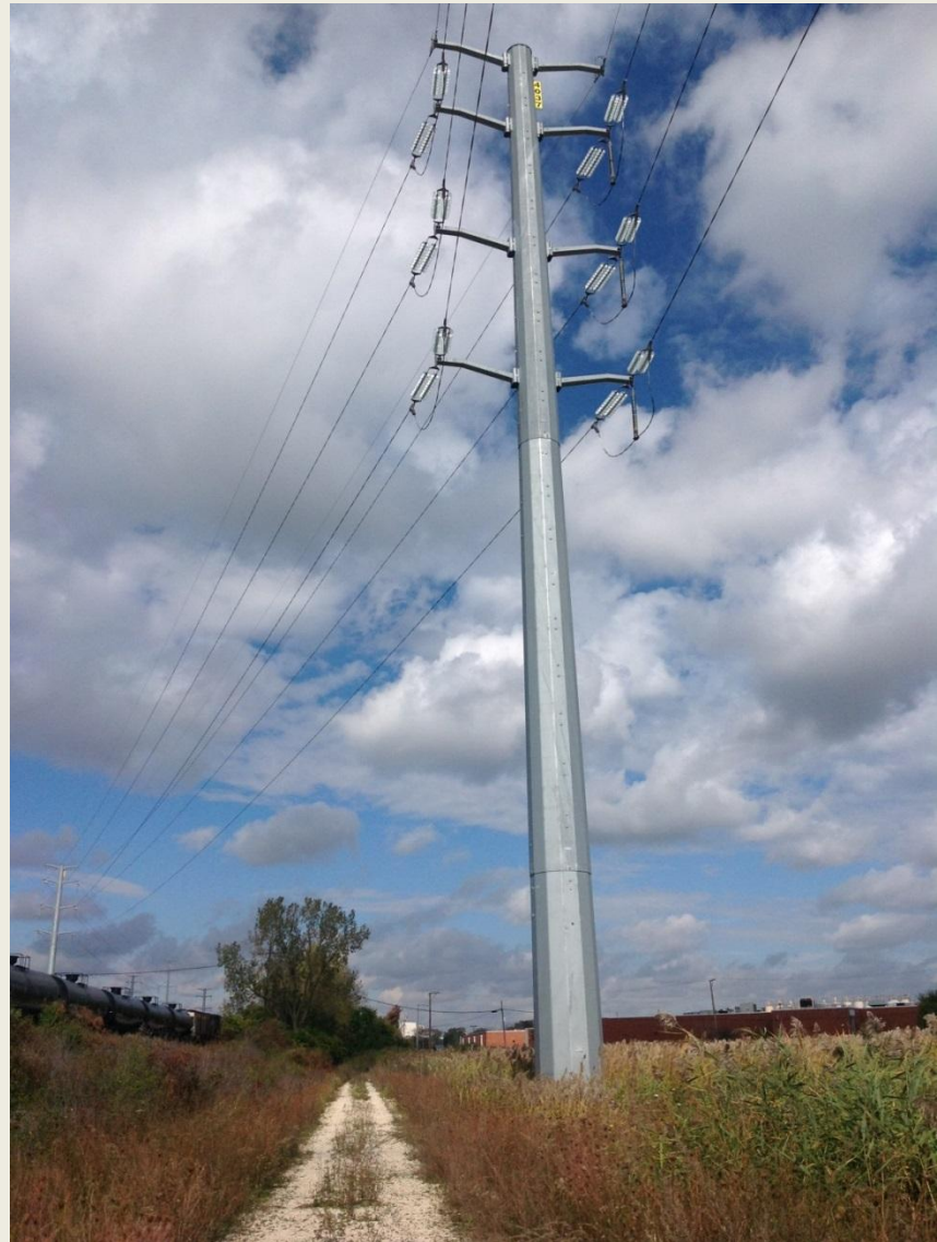
ComEd access road and tower
