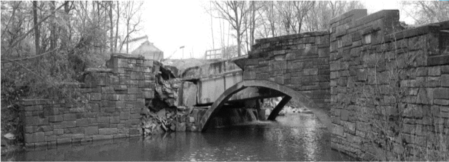
North elevation of aqueduct showing collapse from 2013 flood; taken from HAER report
