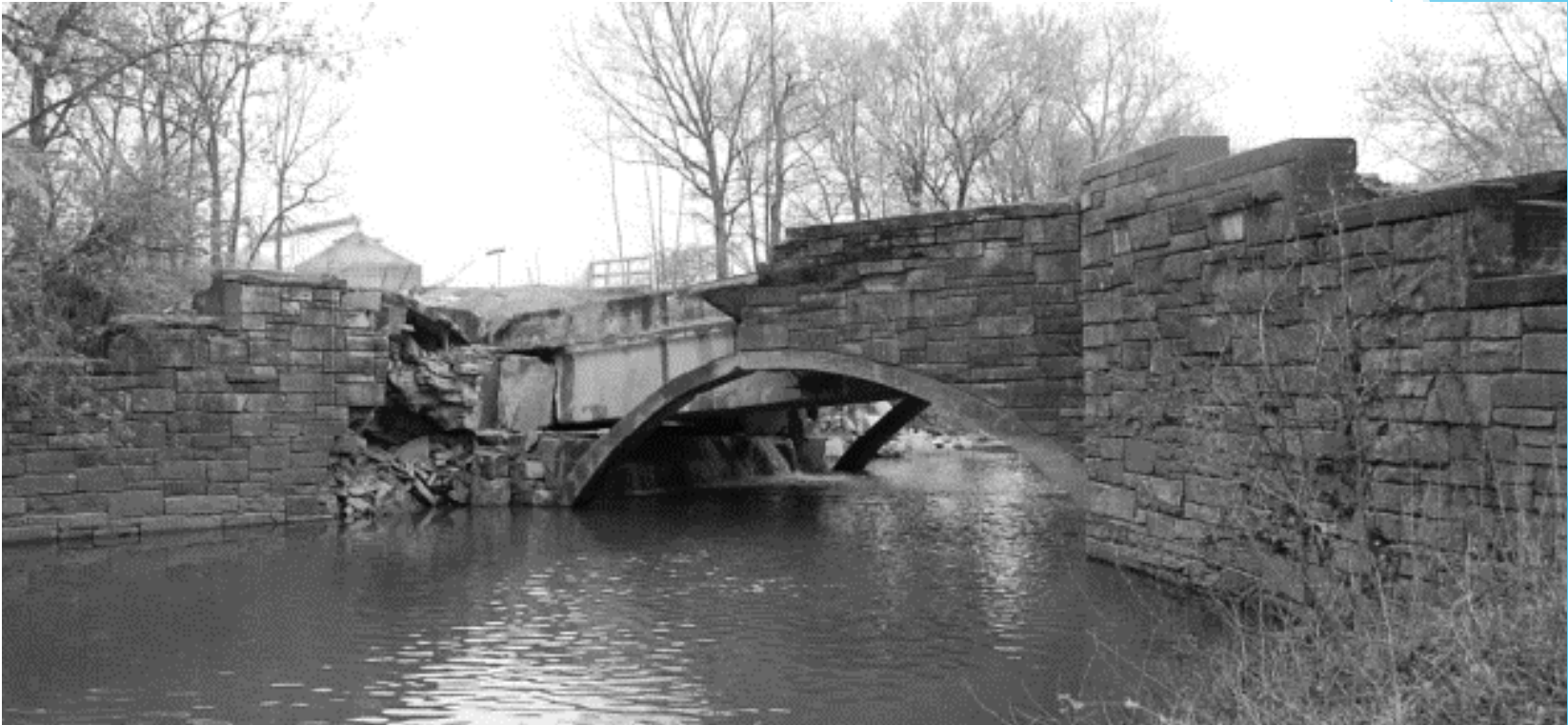
Nettle creek Aqueduct, after 2013 collapse.
