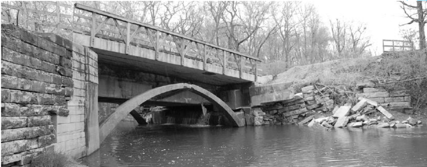
View of the rear side of the northern wing wall of the east abutment after collapse.
