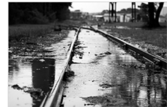
Train tracks partially submerged by excess rainfall.
