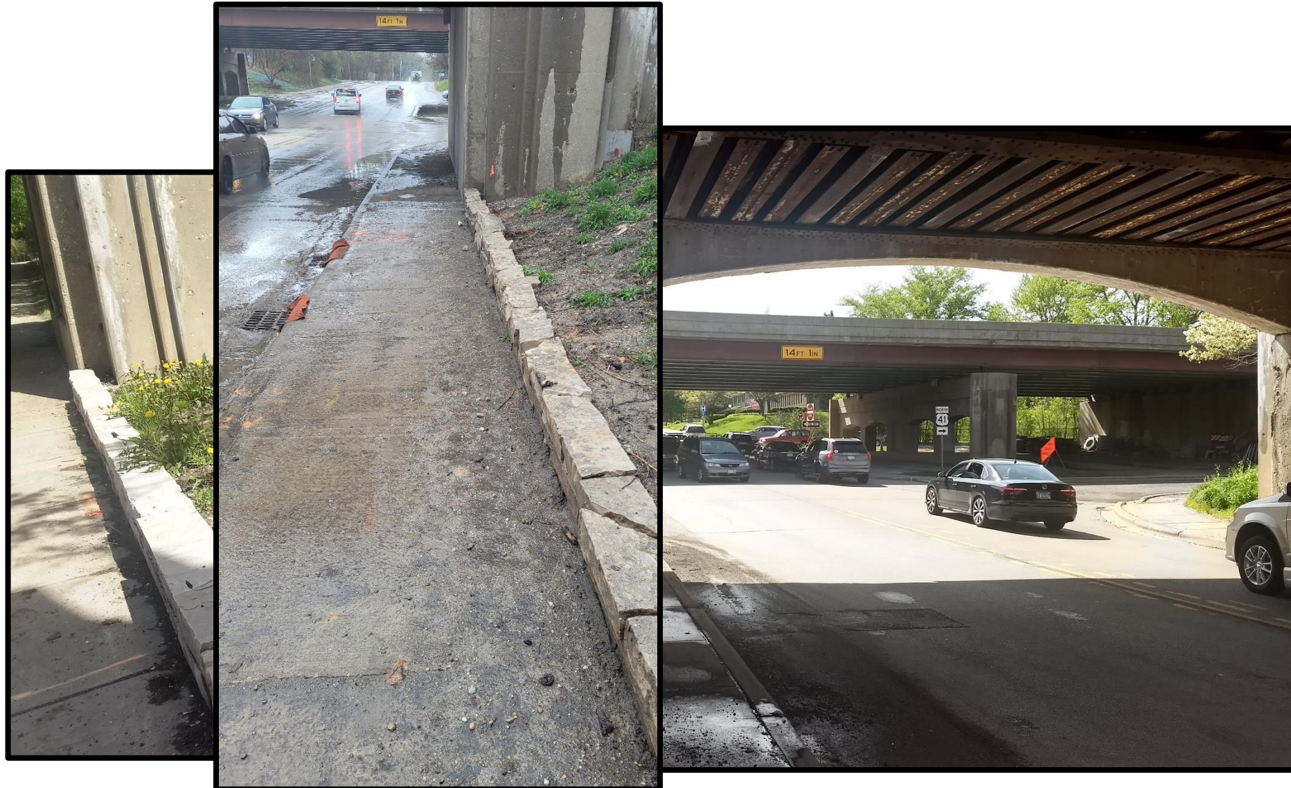
Sediment Washout on Deerpath Road
