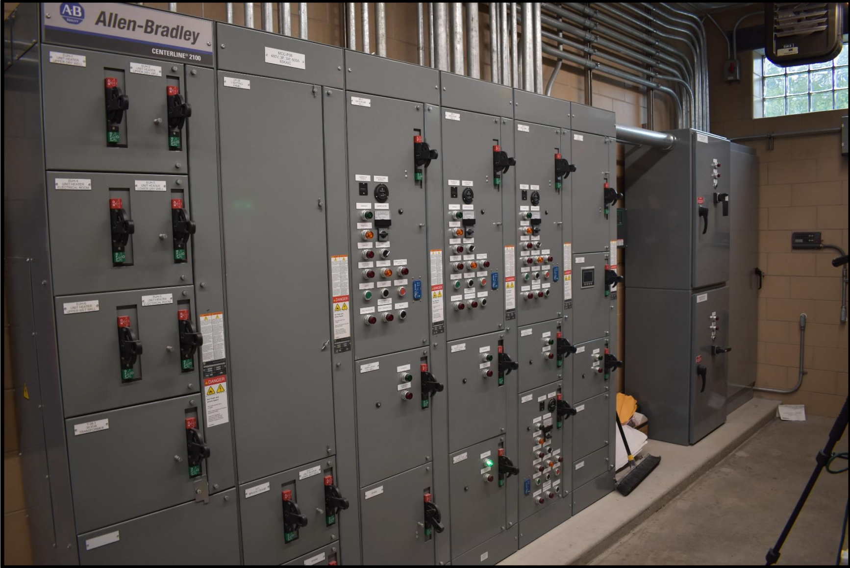
Electric Room SCADA Panel
