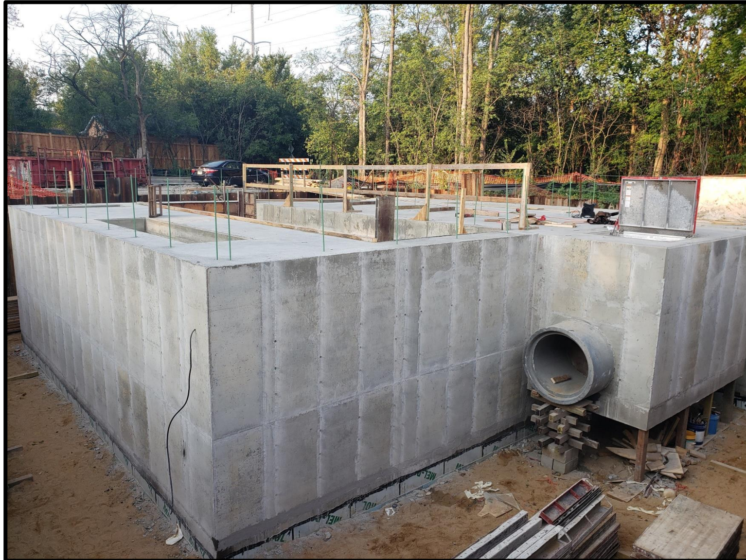
Pump Station Building Foundation and Discharge Chamber Foundation 42' x 39' (Discharge Chamber protrudes 7 feet)
