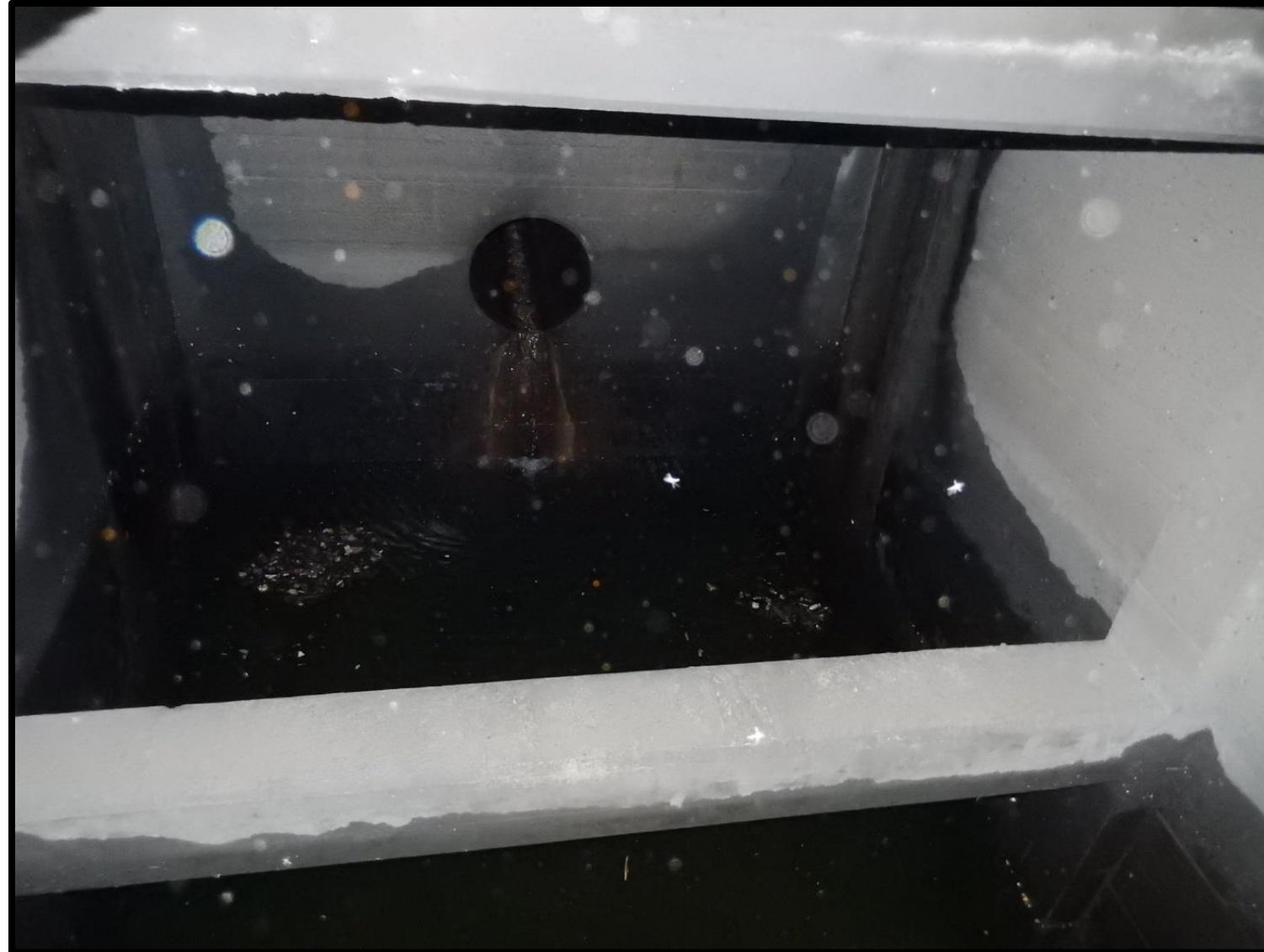
Existing Discharge Chamber 24" outlet pipe, connects to 24"/33" inch bypass sewer which is undersized (10 year capacity, surcharged at 50 year)
