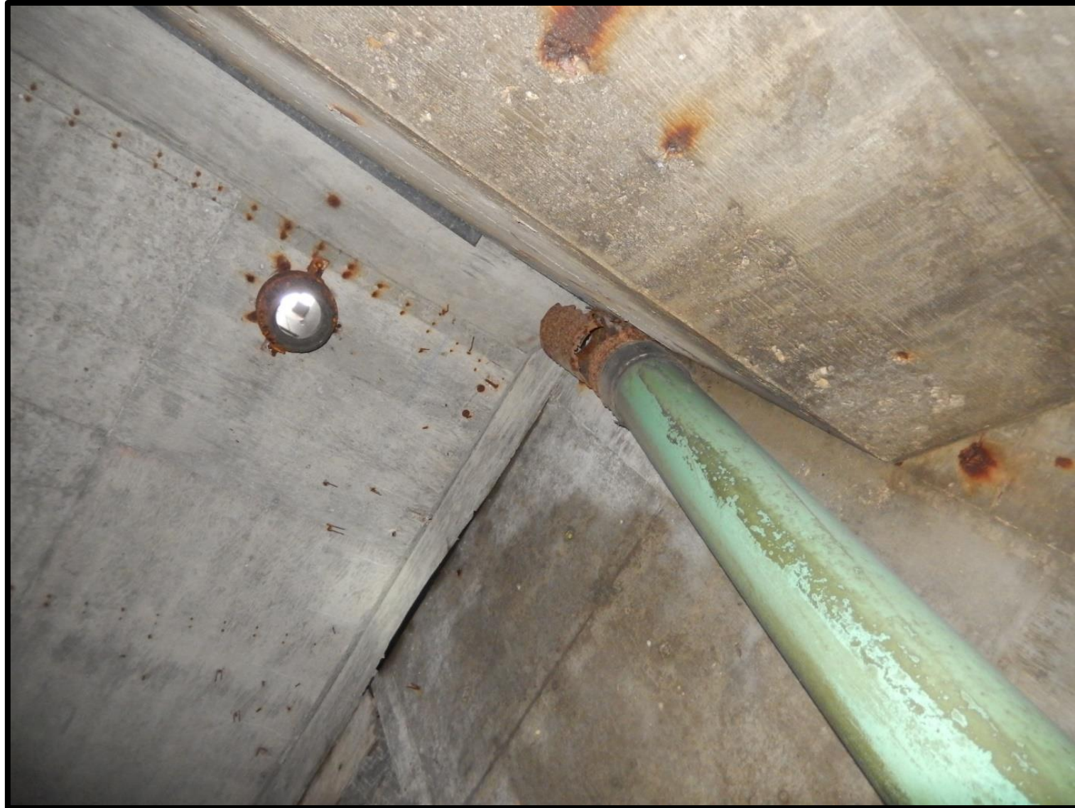
US 41 Scupper Piping Disconnected – Flooding Vault under US 41
