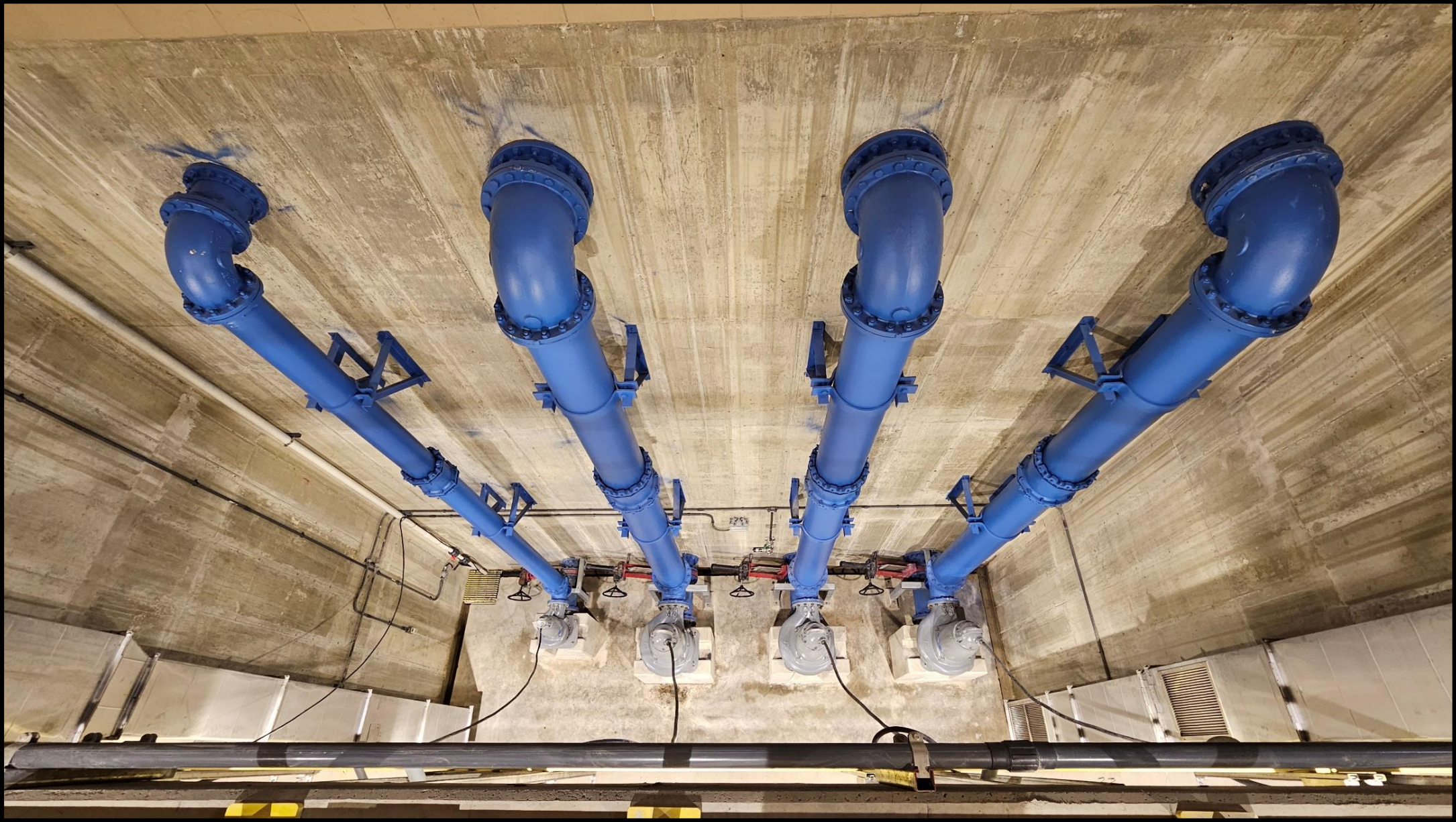
Overhead View of Pumps and Risers
