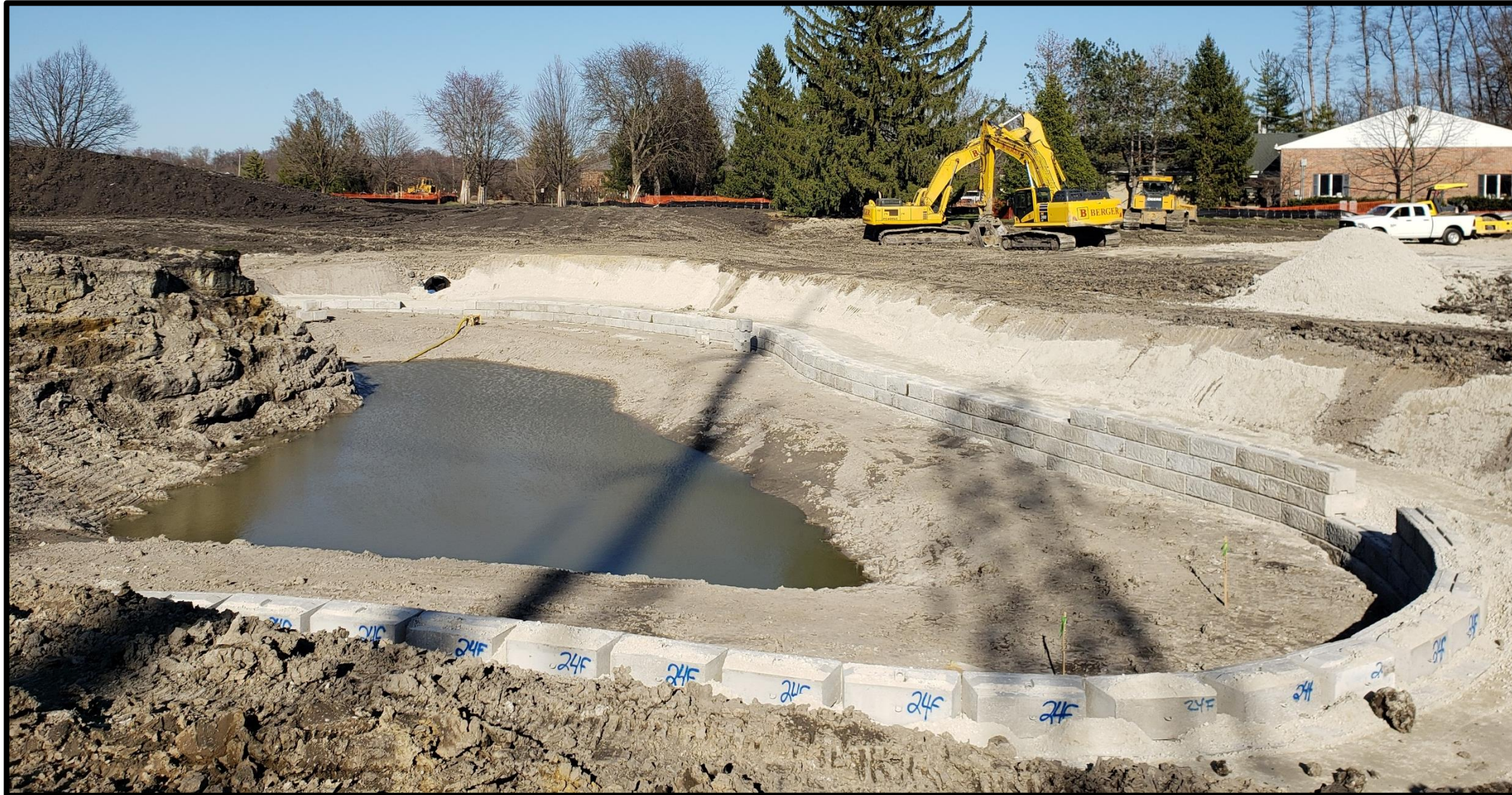
Deerpath Golf Course West Detention Pond Excavation and Retaining Walls 6.05 ac-ft (13.45 ac-ft total)
