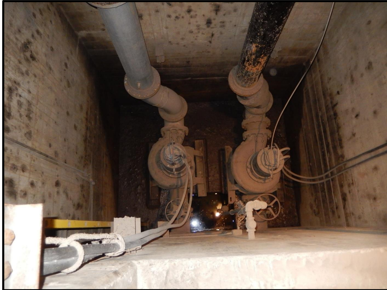
Existing Undersized Pumps 2- 2500 gpm Installed in 1936 (Pump #2 replaced in 1992)
